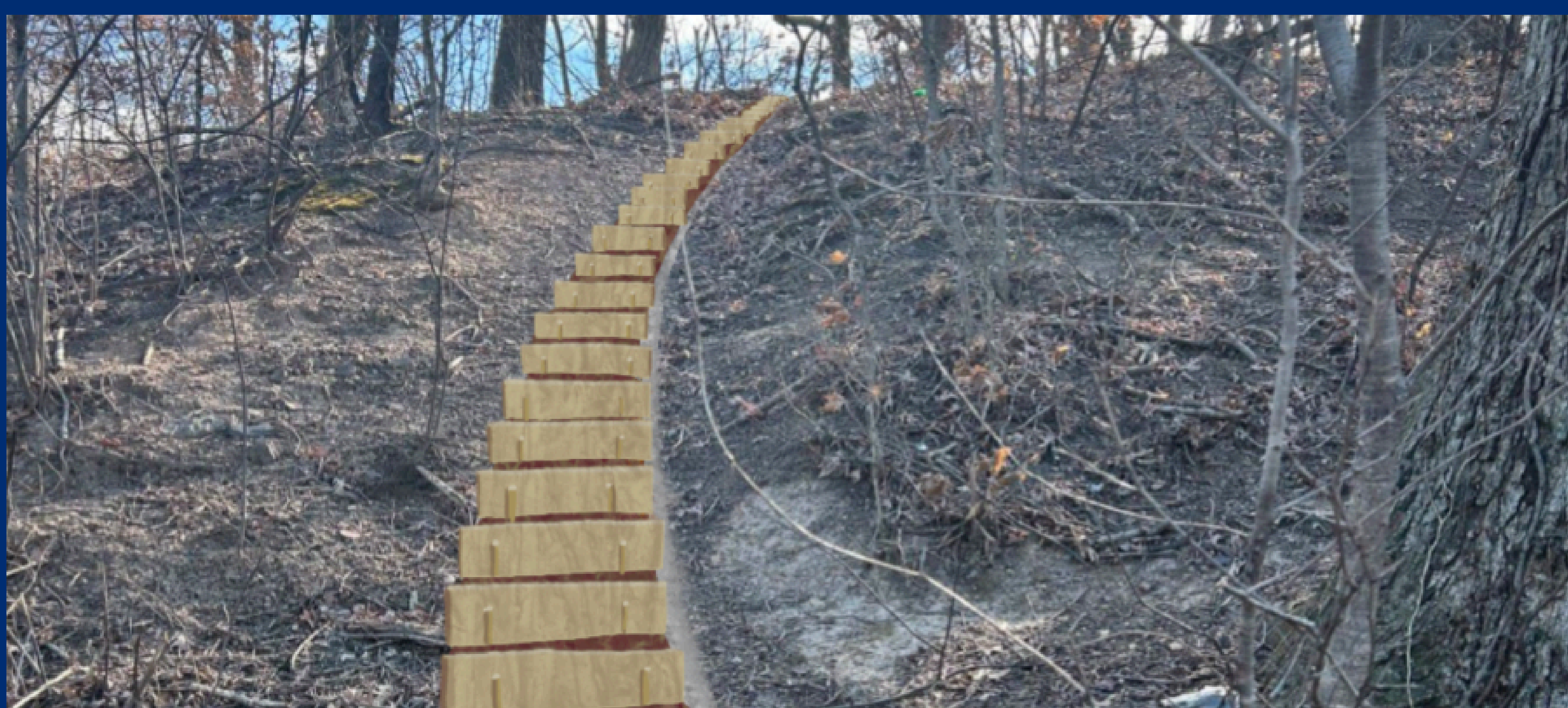
Figure 2: Staircase showing wooden steps, supporting stakes, woodchip treads, and a drainage swale along the hillside.
